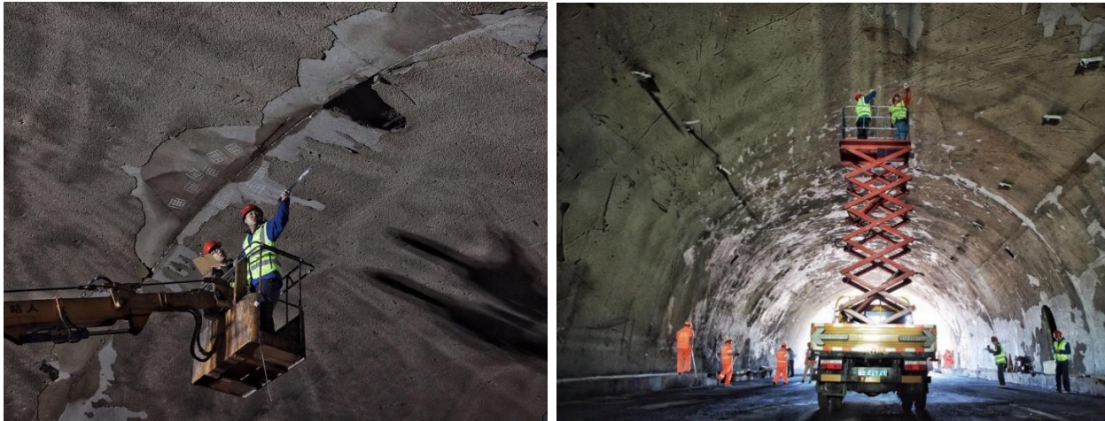
Figure 1: Tunnel lining blast damage(Bjnews 2017)
